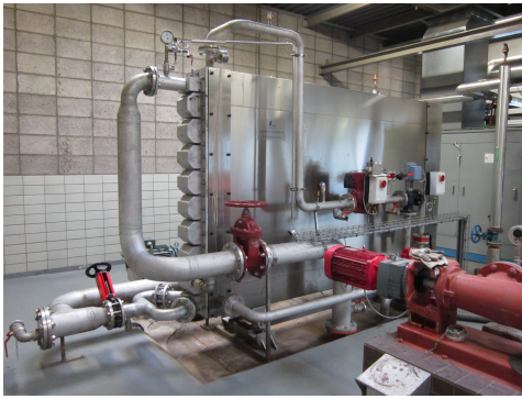
(a) Heat exchanger on the first floor.
