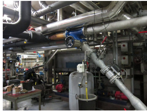
(b) 45 degree junction of primary (lower pipe) and THP sludge (upper pipe).
