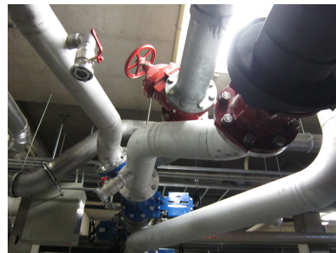
(d) Bottom rear view of the 45 degree junction (middle bottom) of digested sludge (top left) and primary and THP sludge (top right).
