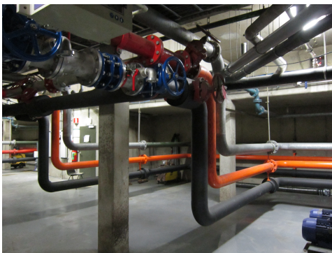
(e) Venturi and pipeline feeding the digester (lower black pipe).
