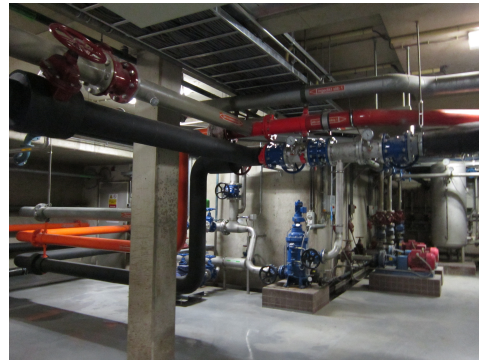
(b) Venturi on the ground floor (lower black pipe).
