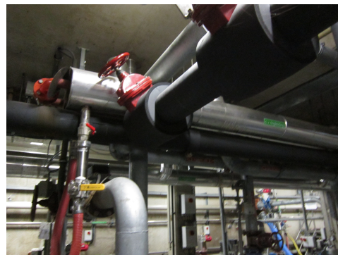
(f) T-junction of primary sludge (left) and THP sludge (right).
