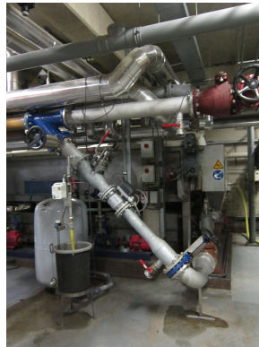
(c) 45 degree junction of primary (lower pipe) and THP sludge (upper pipe).
