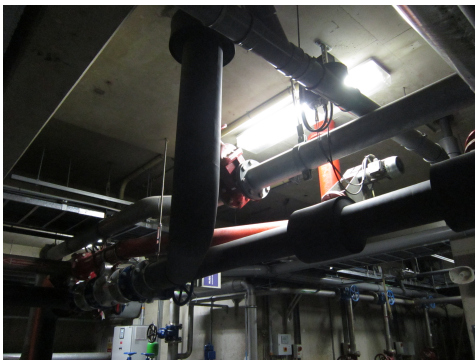
(g) Rear view of the junction of recirculation pipe from first floor (top middle) and THP and primary sludge (right).
