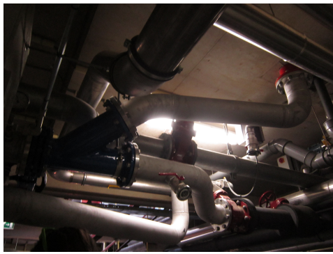
(a) Front side view of the 45 degree junction (left) of primary and THP sludge and digested sludge (top right).
