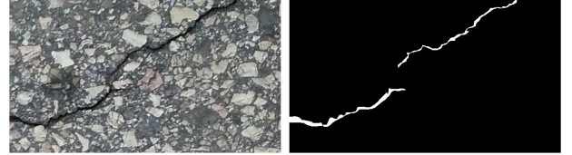
Figure 3. A crack image and the corresponding groundtruth image in CRACK500 dataset
