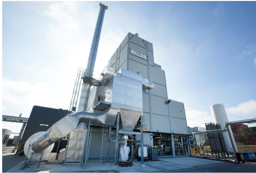
Figure 1.2: BTG-BTL Pyrolysis Plant
