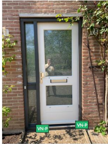
Figure 16: A door with minor wood rot damage (Source: Polyfilla inspection report, 2021)
