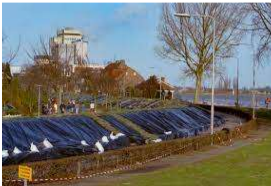
Figure 13 Temporary dike in Kampen ( Destentor.nl, 2021)
