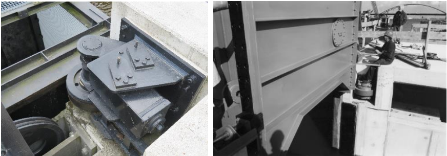
Figure 51. Top guidance Meppelerdiep lock (left) [22], horizontal guidance wheel from rolling gate Nieuwe Oranje lock in Amsterdam (right) [3].
