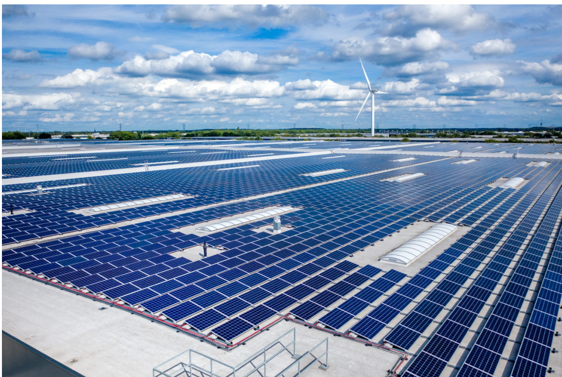
Figure 1.1 One of Sunrock's solar roofs in Tilburg, The Netherlands.
