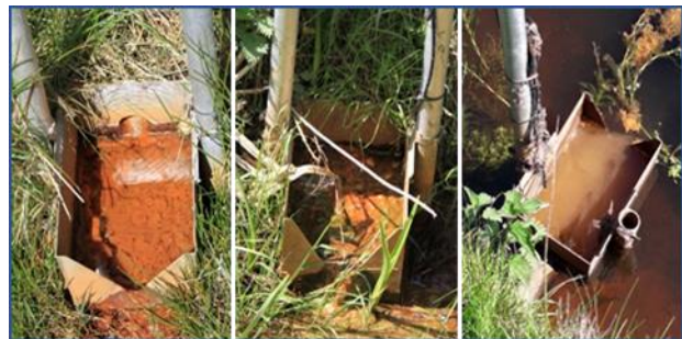
Figure 6: States of the bucket used to measure drain flow. From left to right; as expected, outlet blocked, inundated
