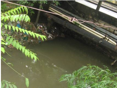
Waste and plastic tubes block water flow at a culvert
