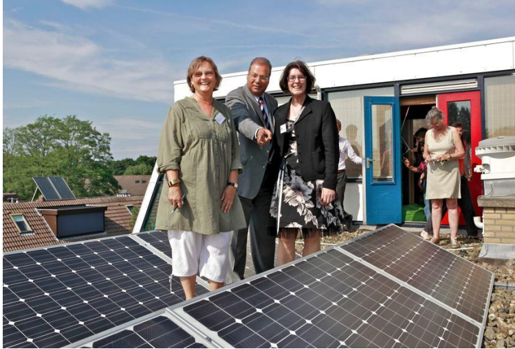
Figure 19 Solar panels installed on the roof of project Houtwijk
