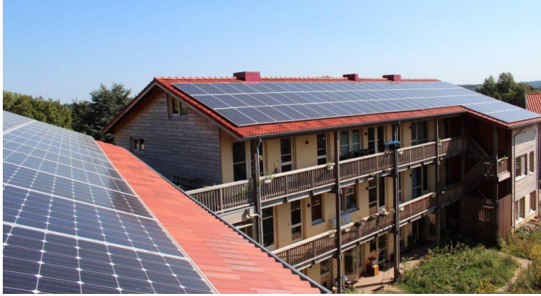
Figure 17 Solar panels installed on the roofs of the houses
