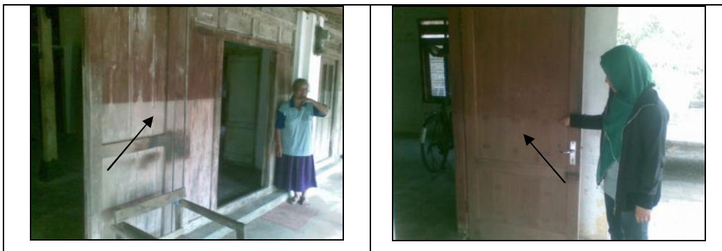
Figure 3-6. Flood marks in desa Kadokan Left : Flood mark in dukuh Nusupan; Right Flood mark in dukuh Kadokan. (Source : Fieldwork 2010).
