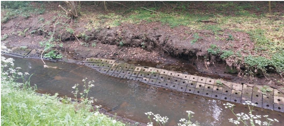
Figure 5: The banks of the Buursebeek, the creek is covered with a geotextile and stones
