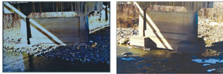
Figure 2-3 Erosion of River Bed at Bridge Abutment (Langer, 2003)
