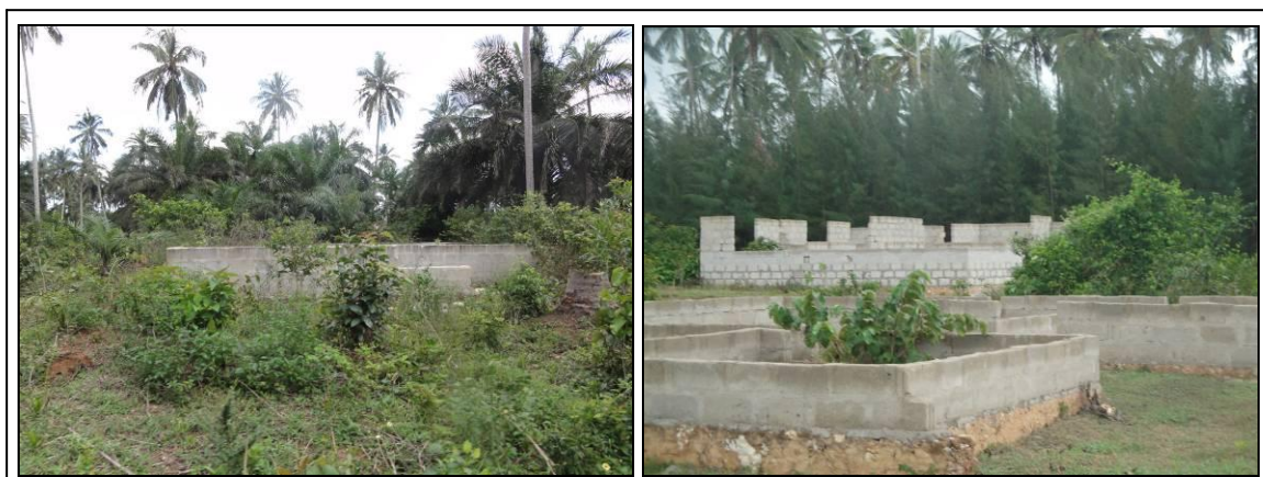
Figure 5-1: Building construction into forest land (Masingini village)
