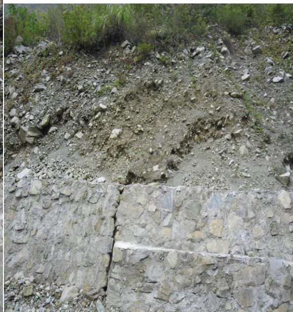
figure 26 shows a broken embankment
