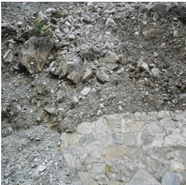
Figure 25 shows over-topped embankment
