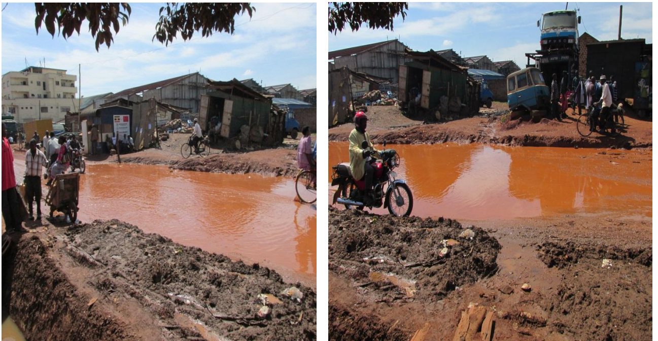
Figure 9: Partially flooded section of the road in the study area
