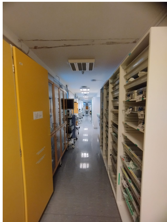
(d) Evacuation hallway, behind the ORs, full with storage. Date: 3 November 2022
