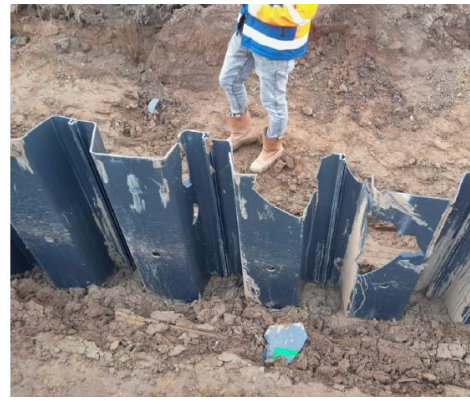
Figure 28. Damage of the upper part of the sheet pile
