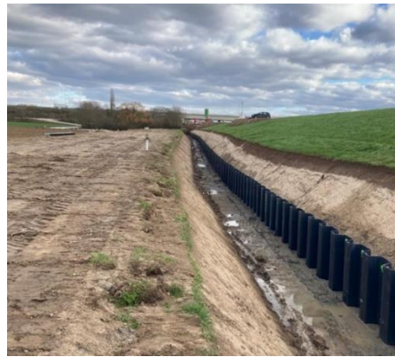
Figure 27. Trench for pile driving is not packed/dense.
