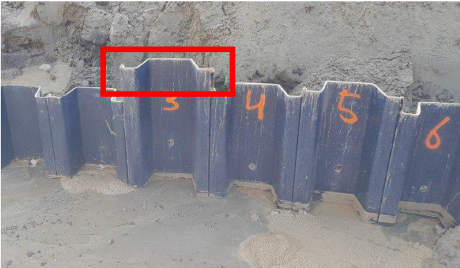
Figure 21. Incorrectly installed sheet pile at project Wolferen Sprok (red box: sheet pile not at required depth).
