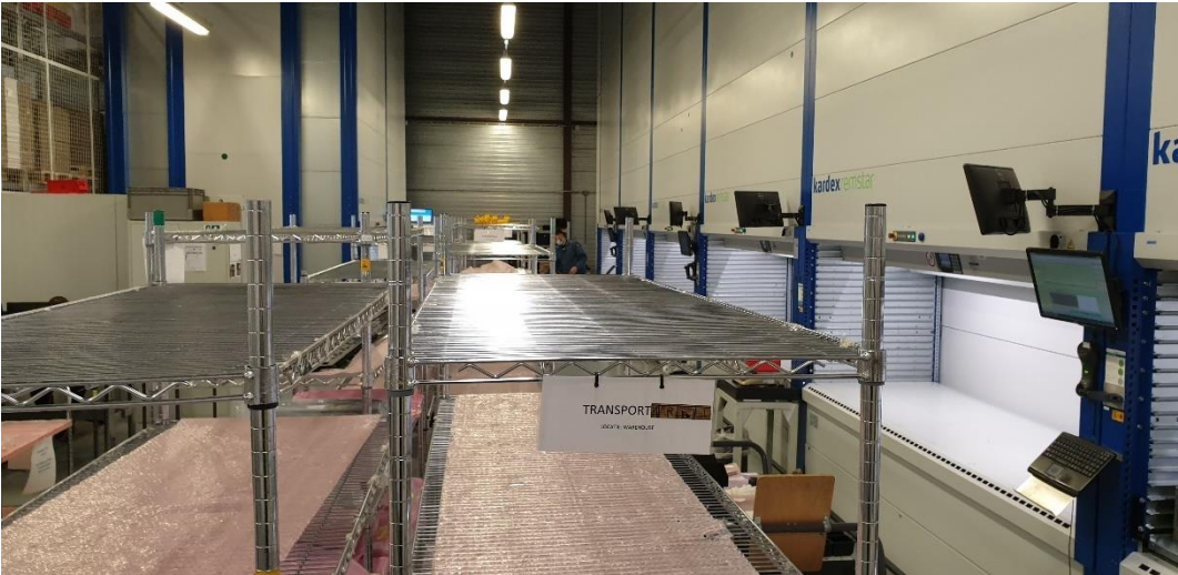
Figure 19 - Overview picture of the ZKDX1001 zone
