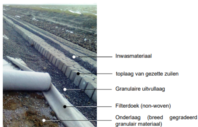
Figure 2.1: Stone revetment during construction [4]. Translation: inwasmateriaal = joint filler / backfill, toplaag van gezette zuilen = top layer of columnar concrete blocks, granulaire uitvullaag = granular layer, filterdoek = filter fabric, onderlaag (breed gegradeerd granulair materiaal) = underlayer (large graded granular material)
