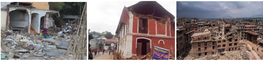
Figure 4.1. Type of openings: damaged walls, roofs, open doors and windows (from left to right)
