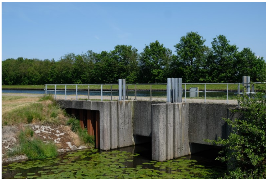
Figure 6: Height difference between Kanaal Almelo-De Haandrik and it's surrounding waterways (Photograph taken by author on 28-5-2023)
