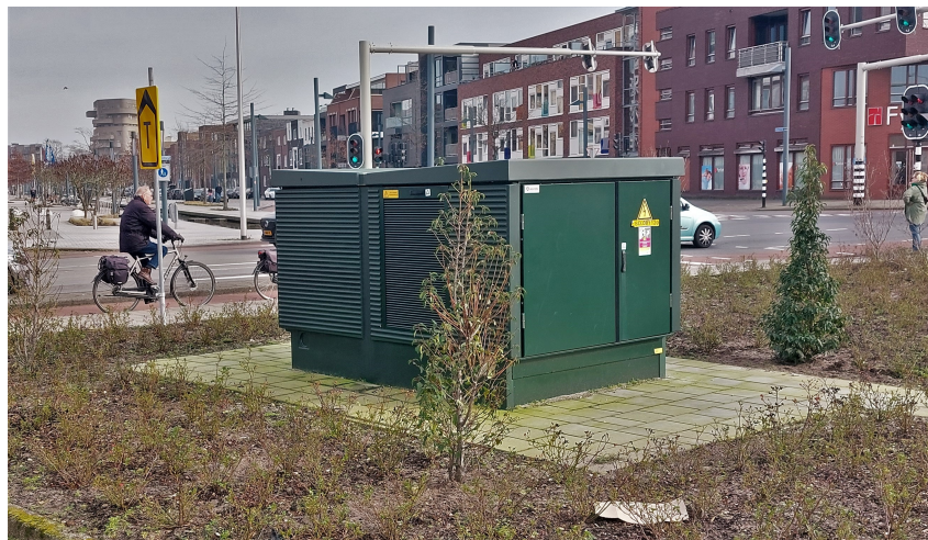
Figure 2.2: Typical modern MV-LV distribution transformer
