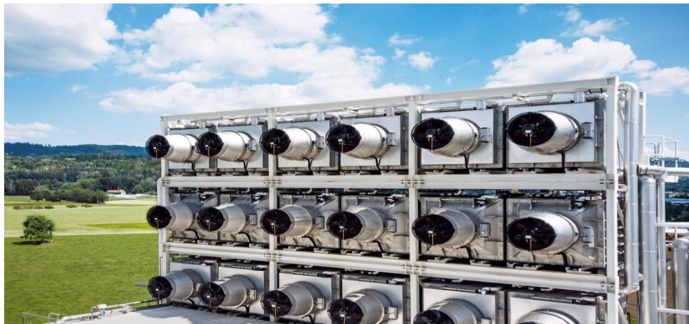
Figure 3: Direct air capture plant in Hinwil, Switzerland ( Gutknecht, 2018 )
