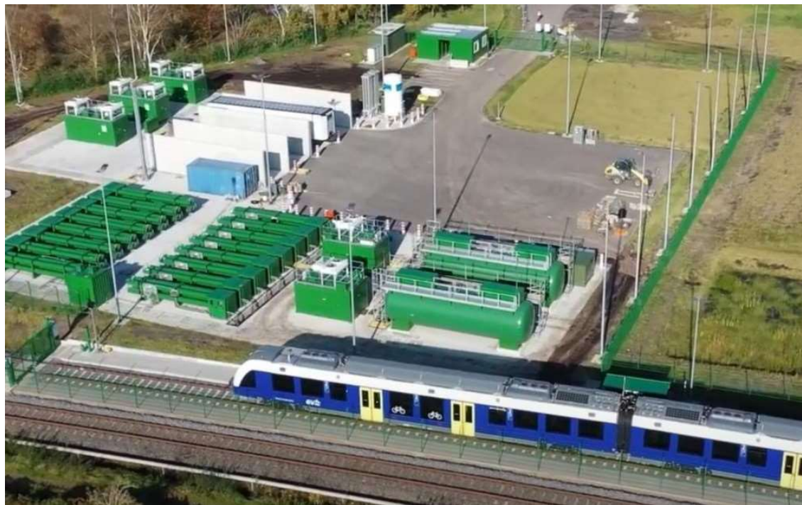
Figure 6 Hydrogen Refuelling Station Bremervörde, image by Linde
