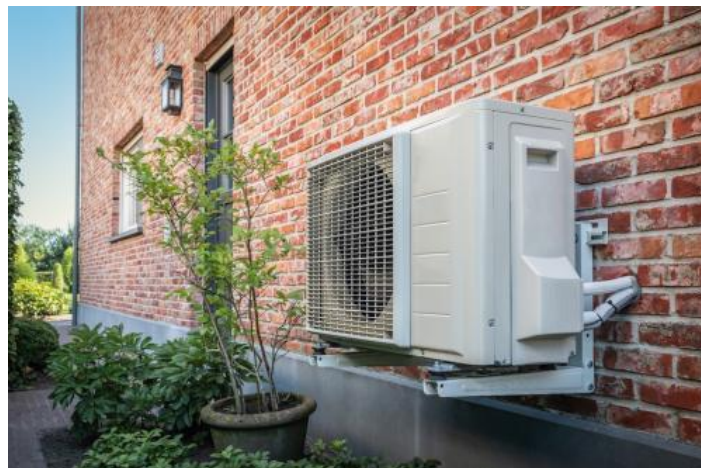
(Outdoor unit of a typical heat pump)
