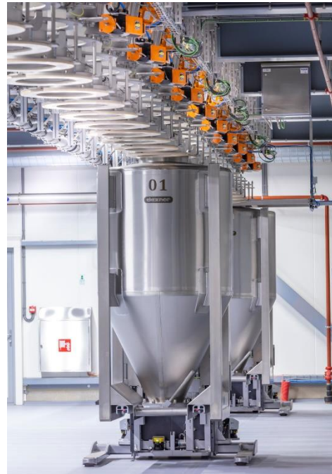
Figure 1.2: An IBC being filled by a hopper of an internal silo.
