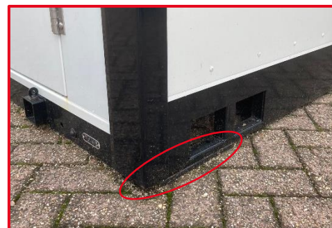
Figure 49 Feet of a Z-box
