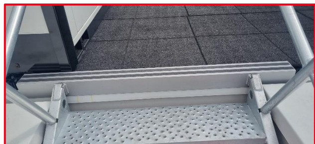
Figure 15: Current L-bracket holding the stairs
