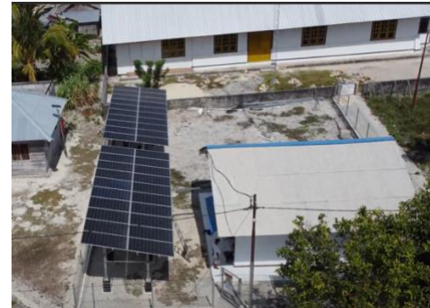
Figure 23. PV Microgrid D in Village D
