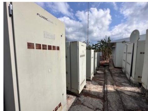
Figure 33. Neglected battery waste from previous project
