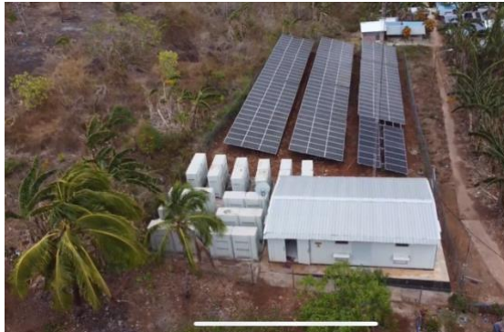
Figure 22. PV Microgrid C in Village C
