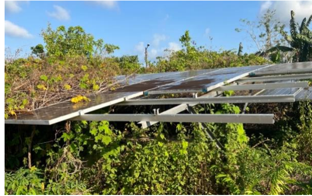
Figure 25. Uncontrolled vegetation and vandalism
