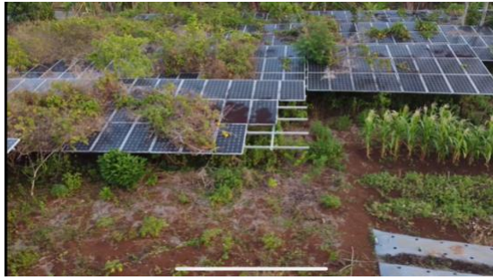
Figure 20. PV Microgrid A in Village A
