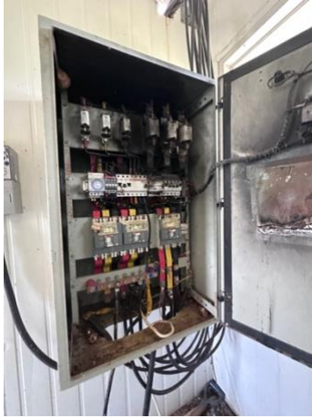
Figure 24. Malfunctioned AC distribution panel
