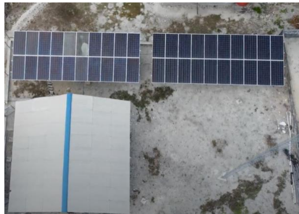
Figure 37. PV-panels of PV Microgrid D
