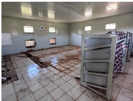
Figure 26. Theft towards battery bank
