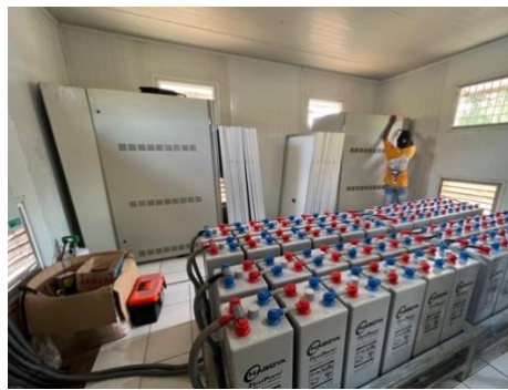
Figure 32. New battery bank
