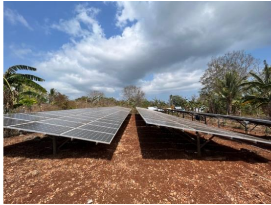
Figure 9: A ground-mounted PV microgrid (Personal Documentation)
