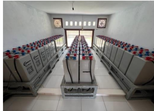
Figure 35. Three battery banks on PV Microgrid D
