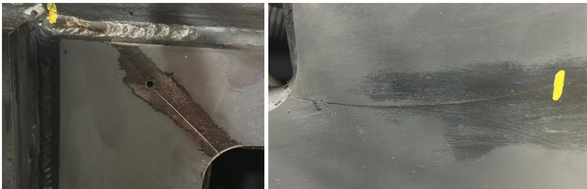
Figure 25, Cracks in the frames
