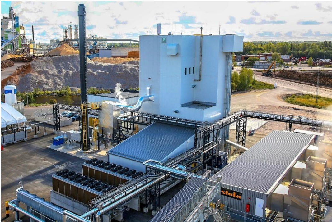
Figure 2. Picture of a commissioned pyrolysis plant
