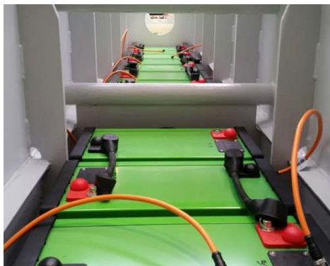
Figure 3 Super B battery set up in electric canal boat [41]
