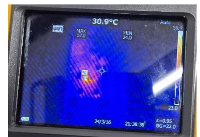
Figure 28 Thermal camera showing temperature increase at snubber
