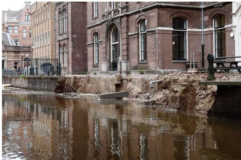
Figure 1 Collapsed quay wall in Amsterdam (source: Herter (2020))
