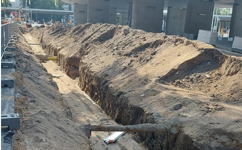
Figure 25: The actual situation during the execution of activity 3 (image taken by ing. J.H. Withaar)
