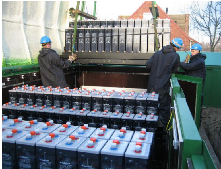
Figure 2.5: A large battery is installed in The Netherlands. (source:Alliander 2 )
