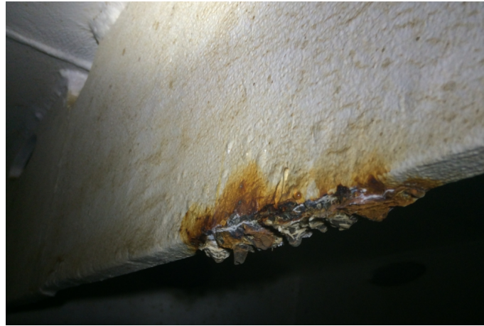
Figure 4.3: Challenging geometry for rust inspection. Image courtesy of Warre te Riet o.g. Scholten.
