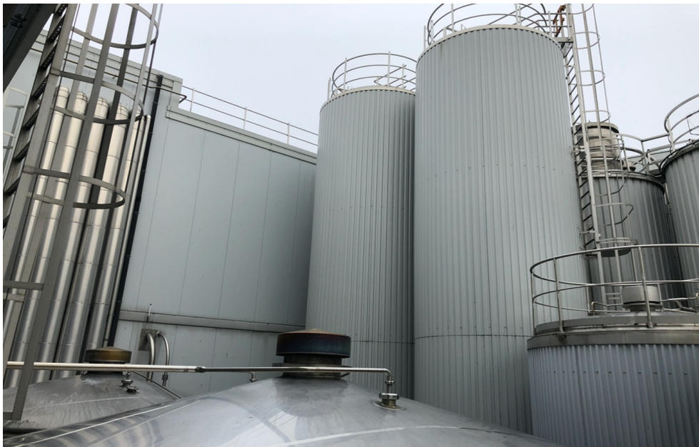
Figure 3: Buffer storage 95KL
