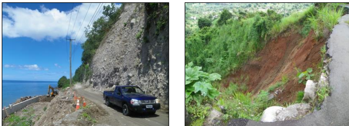
Figure 19. Rockfall and embankment failure in Dominica - Champagne beach area (Left), and Embankment failure in Saint Vincent – Belmont Landslide (Right).
