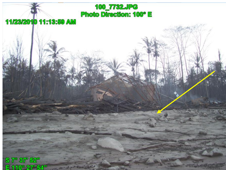
Figure 55. Building that damage by pyroclastic flow and pyroclastic surge (Photo source: BPBD Sleman)
