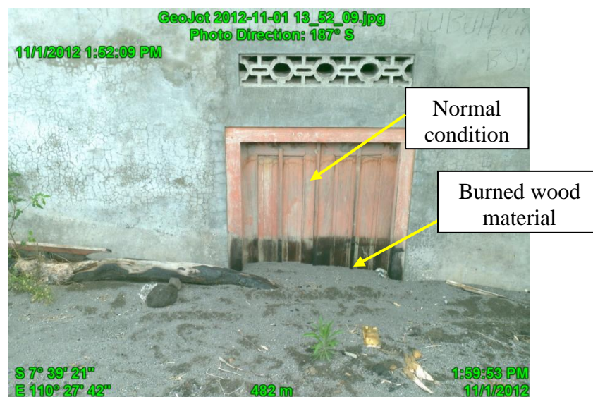
Figure 56. Building that damage by pyroclastic flow with lower intensity
