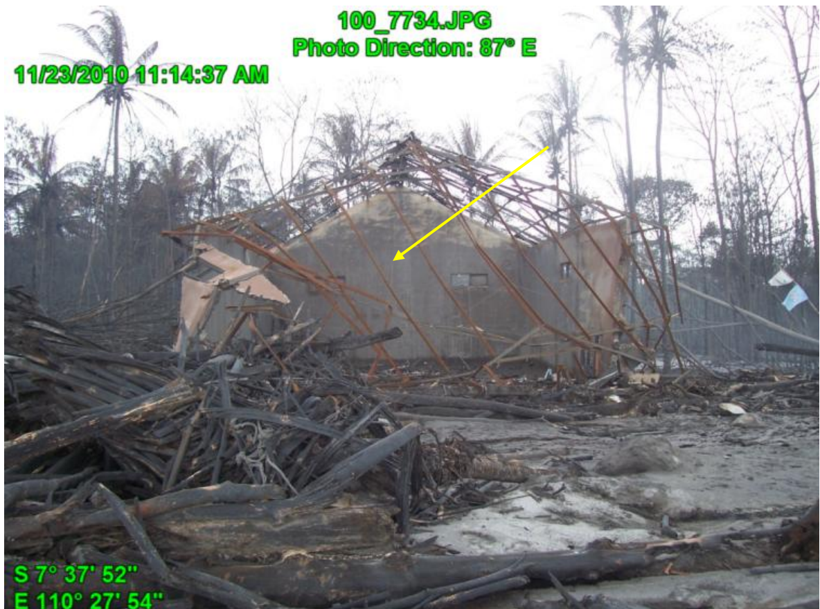
Figure 57. Building that damage by pyroclastic surge (Photo source: BPBD Sleman)
