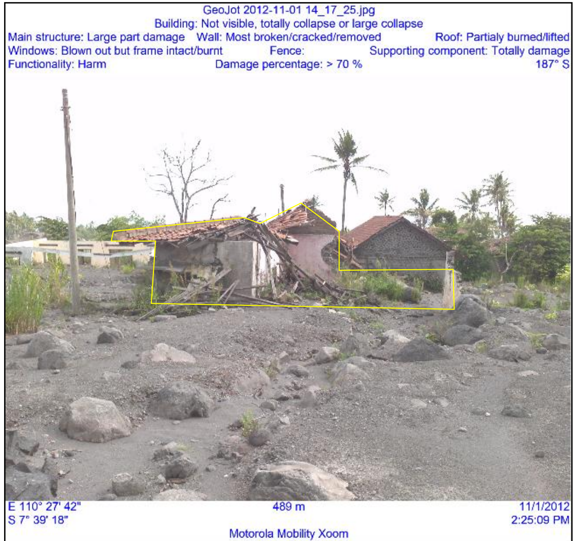
Figure 52. Building damage interpretation sample (direction of 187 ° S)
