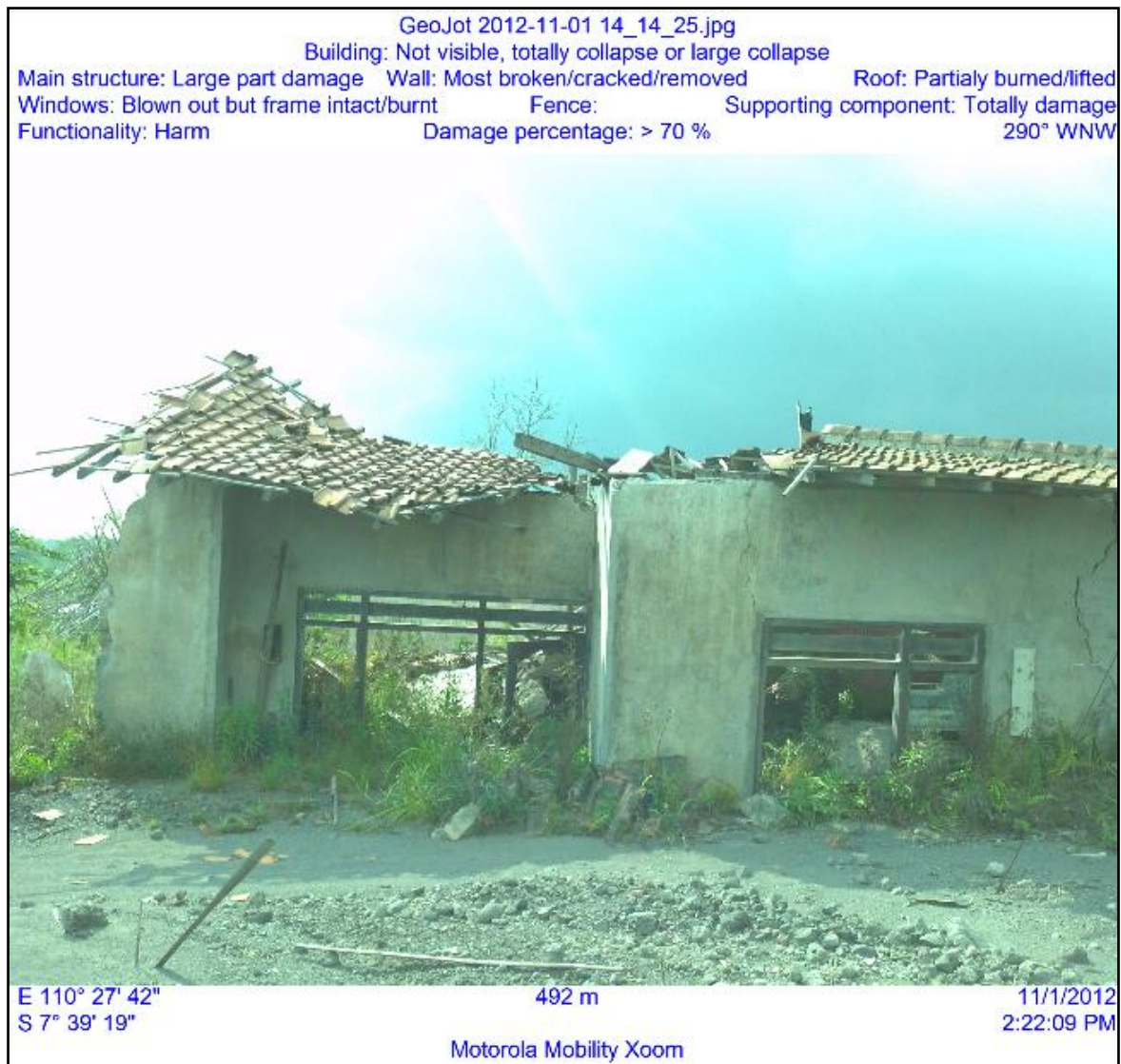
Figure 51. Building damage interpretation report from Geojot to GPS Photo Link (direction of 290 ° WNW)
