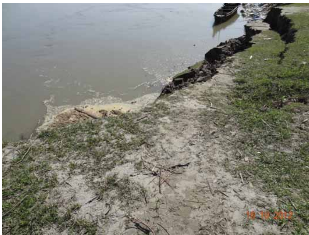
Figure 7.2: Active riverbank erosion process at Salmora
