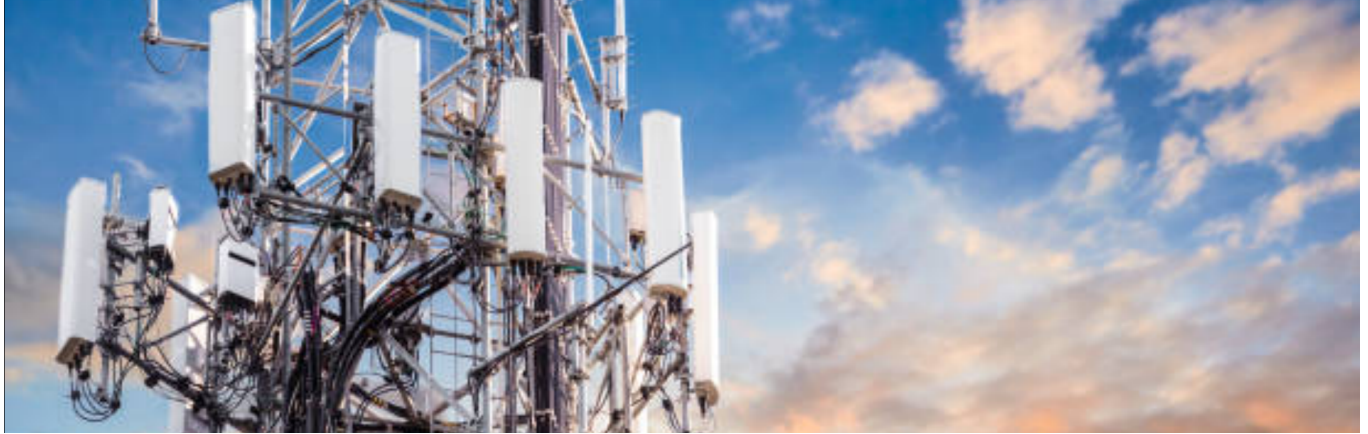
Fig. 1. Transmitters on a base station
